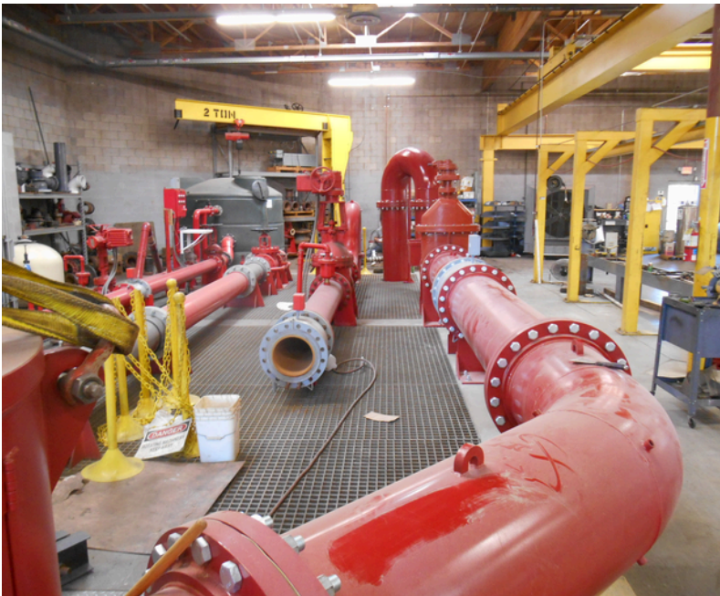
National Pump Test stand where the pumps were tested
